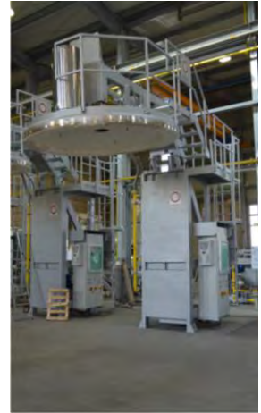
Ladle preheating burner
