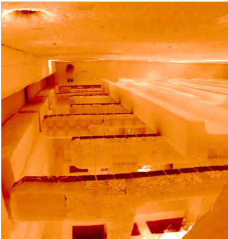
Grey Mill reheating furnace, soaking zone
